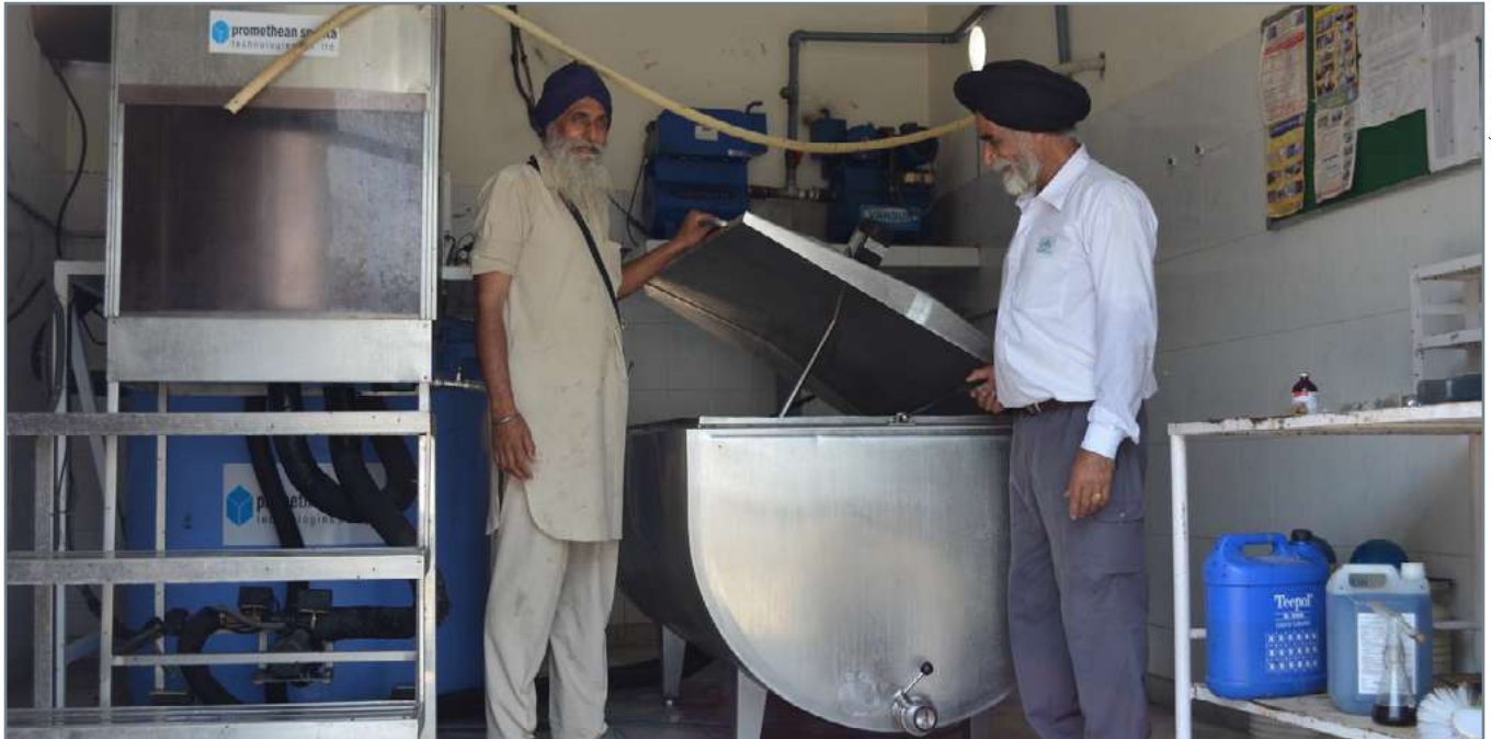
1,000 litre Rapid Milk Chiller installed in Moga (Punjab, 2014)
