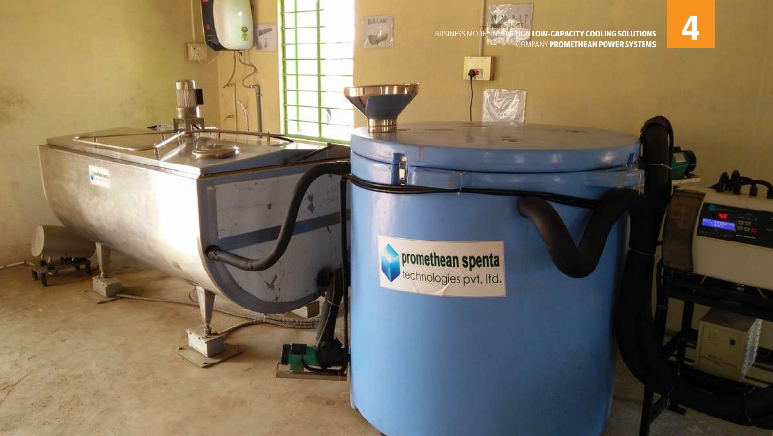
1,000 litre bulk milk cooler installed in Dharmapuri (Tamil Nadu, 2016)
