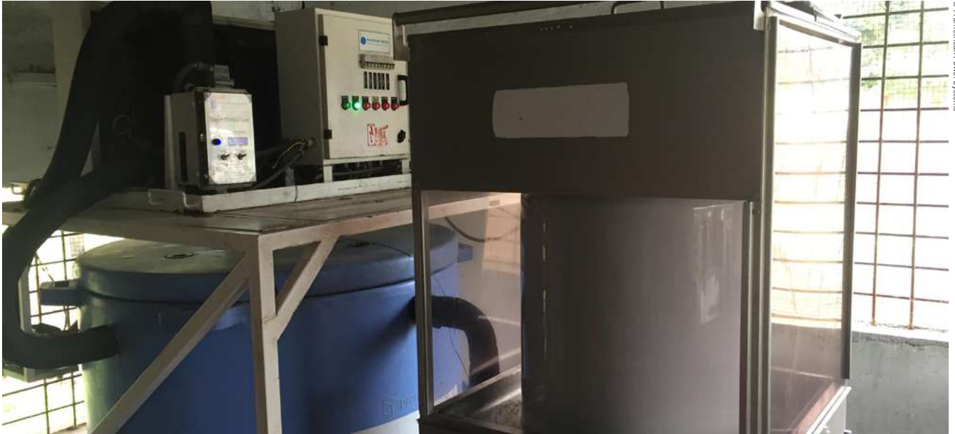
First Rapid Milk Chiller installed at Virar (Maharashtra, 2013)
