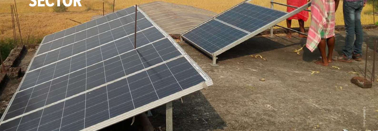
Beneficiaries and Resham Sutra's team members inspecting the installation of solar panels for community silk reeling shed in Ramgarh (Jharkhand 2016)
