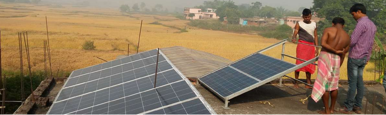
Beneficiaries and Resham Sutra's team members inspecting the installation of solar panels for community silk reeling shed in Ramgarh (Jharkhand 2016)
