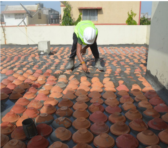
Figure 12. Installation of inverted earthen pots in India. Source: Mansi Shah demonstration project
