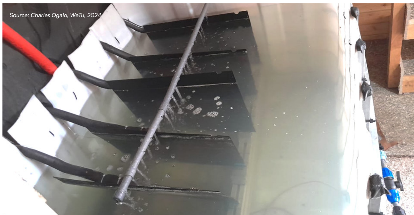
Figure 35. Cooling units with evaporator plates immersed in a water chiller
