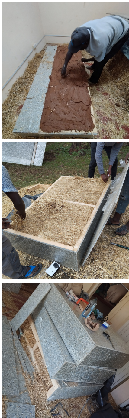
Figure 14. Clay trial (top), filling up insulation panels tightly with more straw (middle), and completed panels ready for assembly (bottom)
