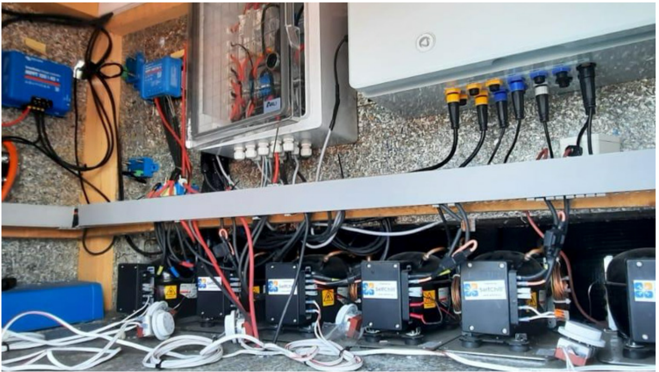
Figure 63. Installed low-carbon cold room (inside and outside) including the technical room with compressors and other electrical equipment
