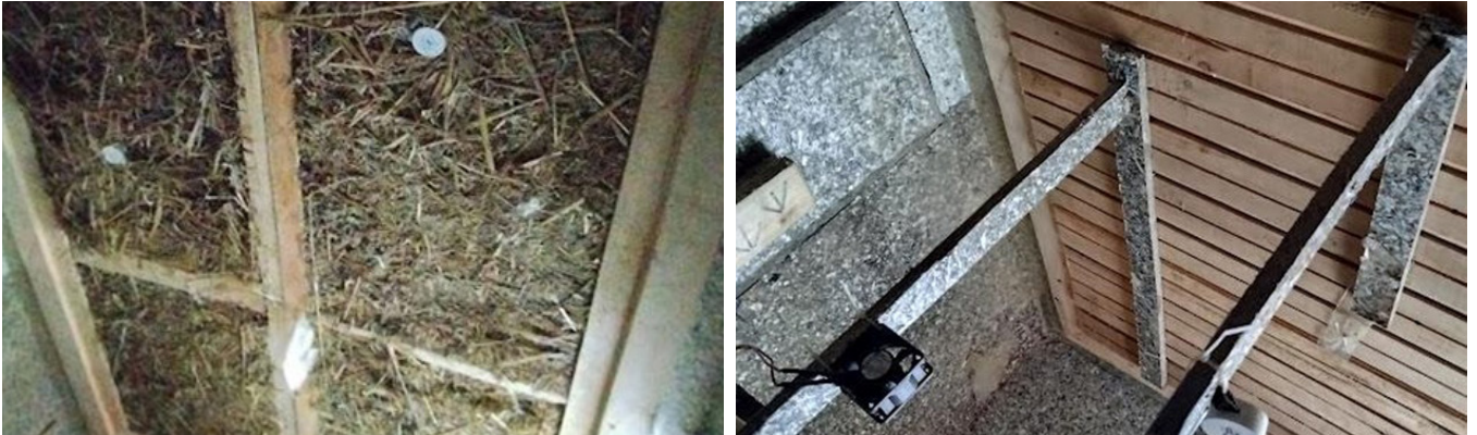
Figure 20. Replacement of eco-boards with T&G timber to protect straw bales from high humidity
