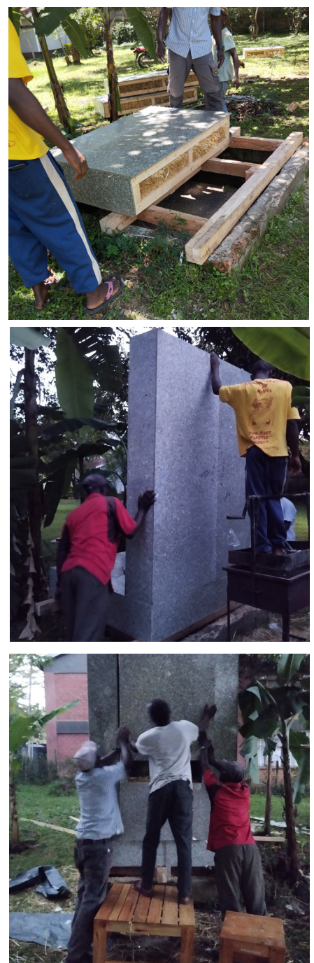
Figure 15. The assembly of the mock-up cold room
