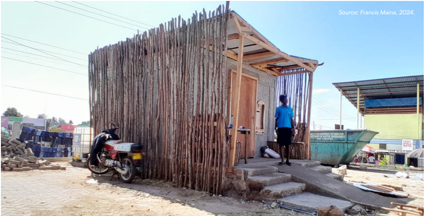
Figure 64. Final low-carbon cold room installation in the Homa Bay market, Western Kenya
