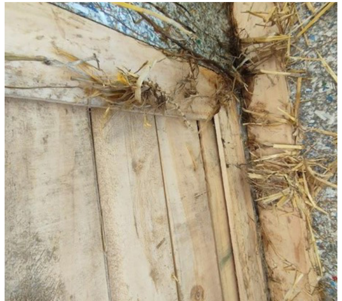
Figure 21. An eco-board insulation panel with damp straw identified during the trial (top), and dry straw with clay plaster (bottom)
