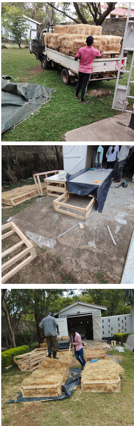
Figure 13. Straw bales delivery to site (top), timber frame fabrication (middle), and straw bale compaction into the insulation panels (bottom)
