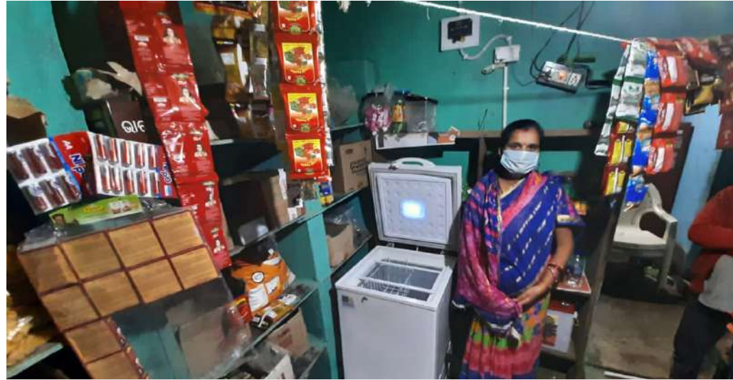
DDSR 100 L is installed at Bhawanipatna, Orissa through our ground partner DAPTA
