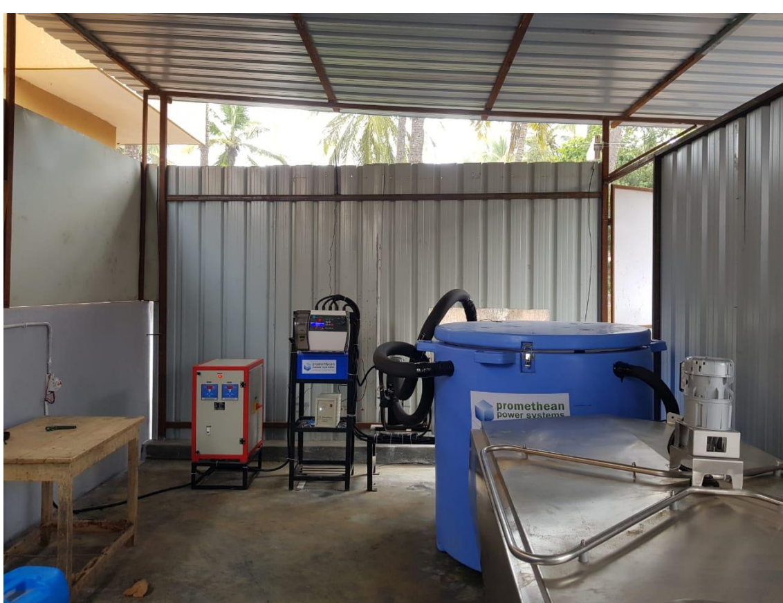
1000L Milk Chiller With Thermal Storage System and Remote Monitoring at a site in Karnataka, India Credit - Promethean Power Systems
