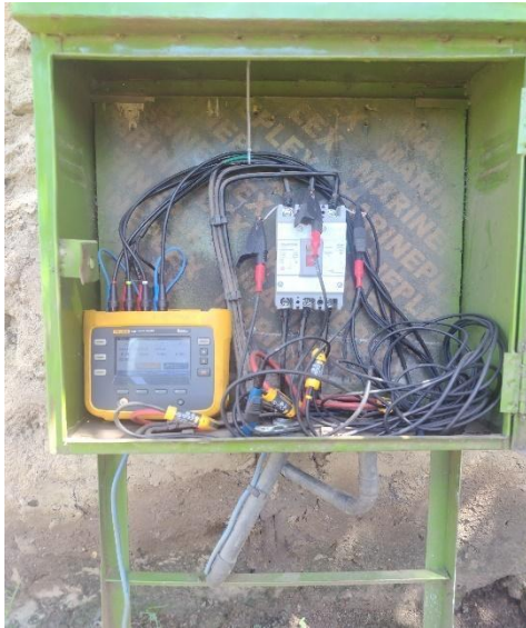
Figure 14: Fluke 1736 Installed at the Main Incomer of Customer #1's Milling Machine
