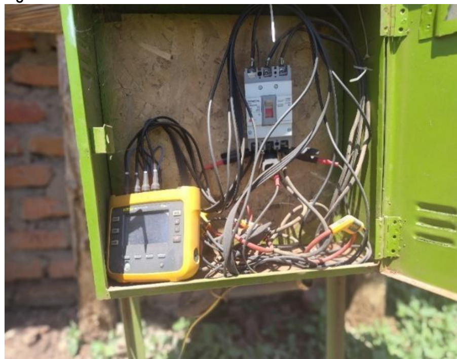
Figure 20: Fluke 1736 Installed at the Main Incomer of Customer #2's Milling Machine
