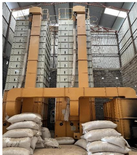
Image 10B: Electric drying units at MRGM
