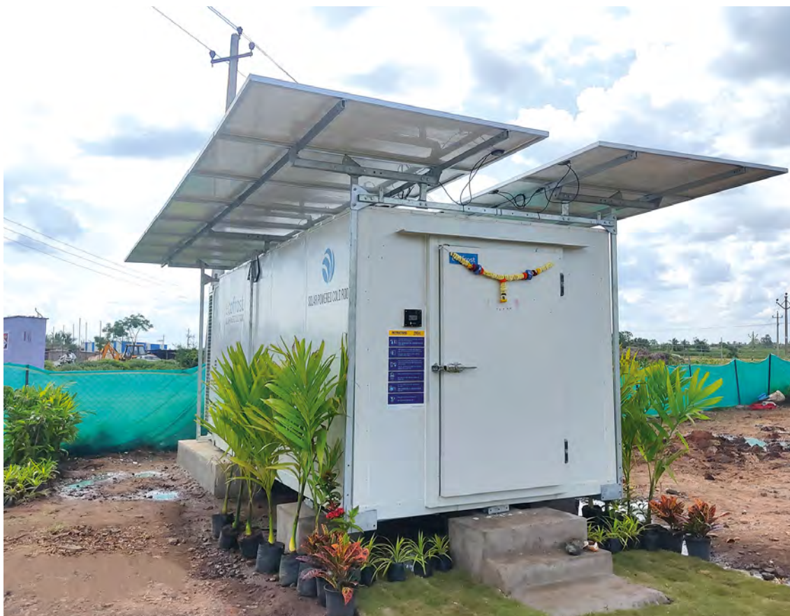
Figure 5.14 Attached solar array ( Ecofrost ).
