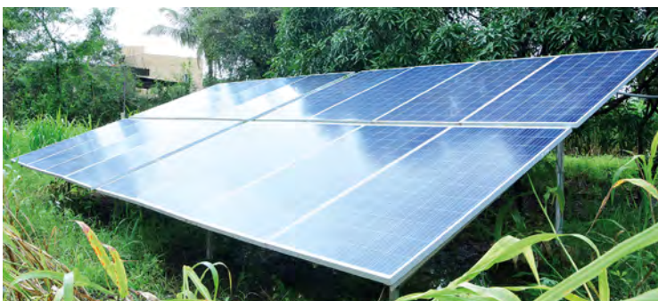
Figure 5.9 Array of solar PV modules (Promethean).
