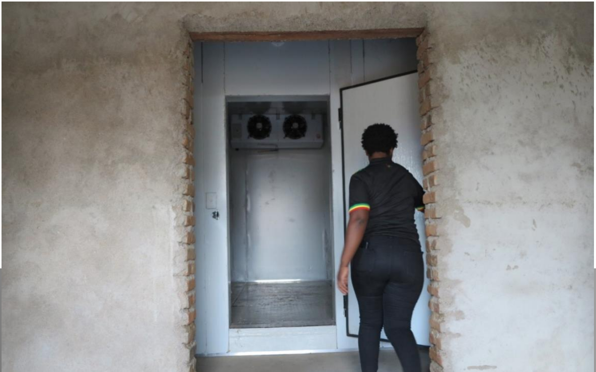
Photo 1. Newly constructed building in Rumphi, northern Malawi containing a low cost “flat pack” cold room powered by solar energy and an area for receiving, sorting and selling
