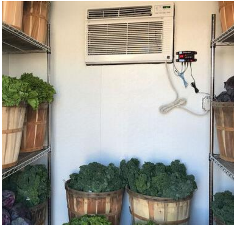
Photo 4. Cold room utilizing an inexpensive window air conditioner with a CoolBot controller
