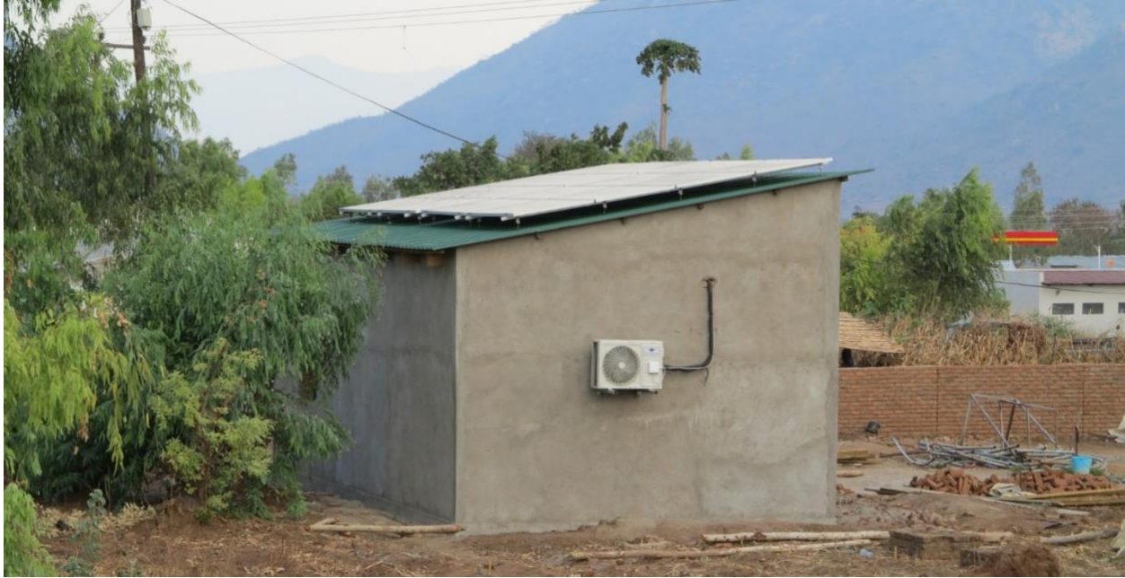
Photo 5. Another view of the multi-purpose building and solar powered cold room in Rumphi, Malawi
