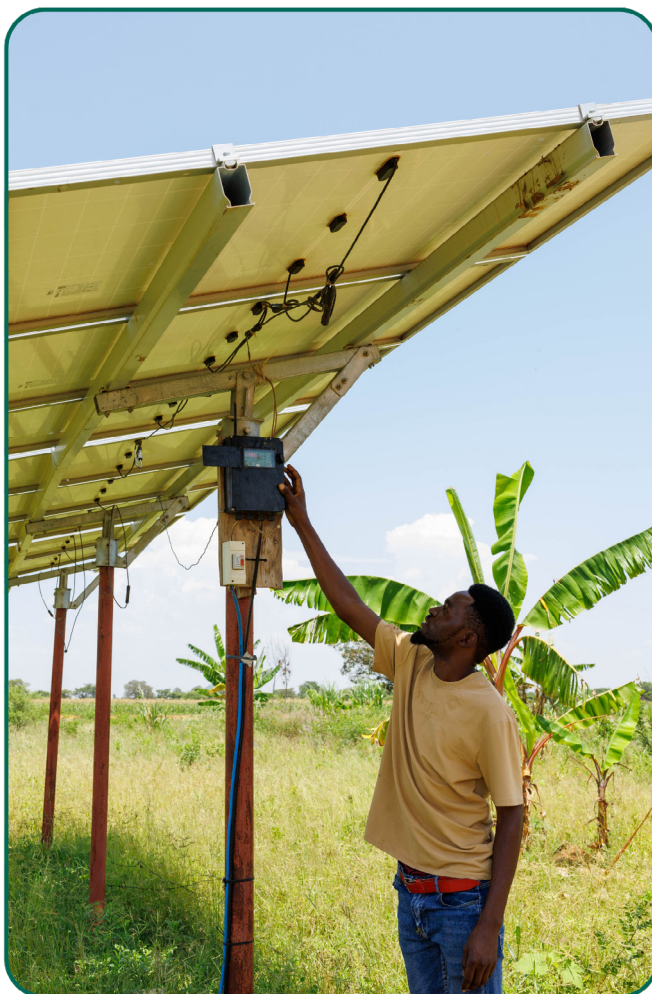
Remote monitoring boxes can be maintained manually, such as this one beneath a solar water pump
